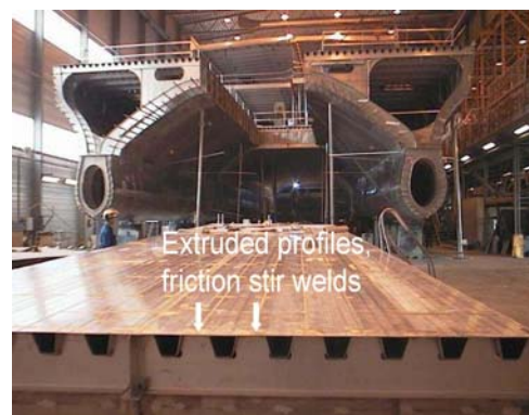
Fig. 10 Fabrication of high speed craft by using extended panels joined by friction stir welding
