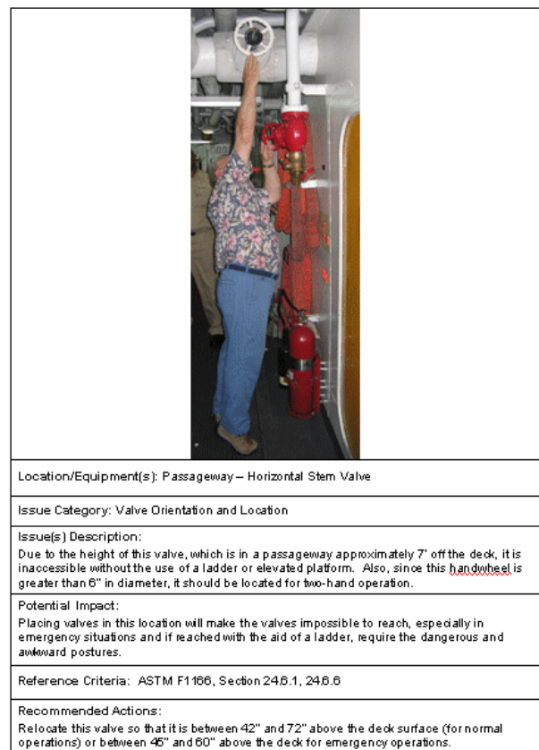
FIGURE 1. Valve Orientation and Location: Main Passageway
